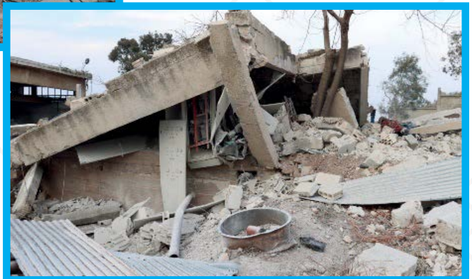
Station structures with damage.
