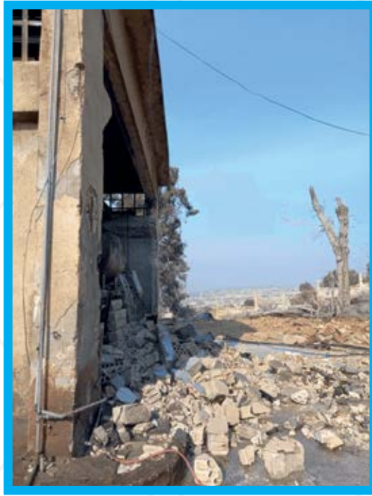
After the assault, the eastern façade of Plant 1 at the water station.
